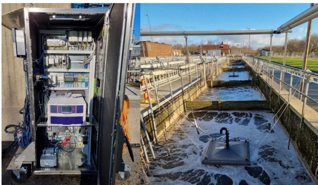
Figure 1. Installed floating hoods and associated measurement equipment at the Klagshamn wastewater treatment plant , south of Malmö.
